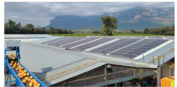
Source: Camco. A solar installation for Eden Fruit, a prominent citrus producer in South Africa.
