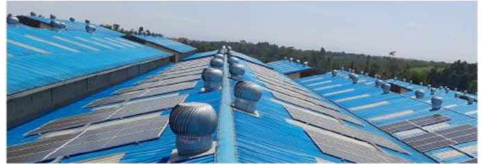
A 90kWp solar rooftop installation provides clean and reliable energy to a large and longstanding printing business near Nairobi, Kenya.
