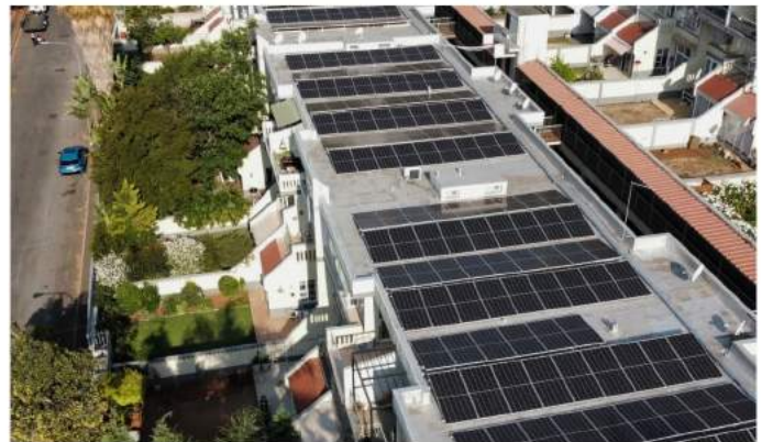
A new rooftop solar PV and battery storage system provides energy to tenants of a 54-unit apartment block in Johannesburg, South Africa
