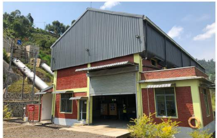
Penstock and Powerhouse: end of channel water is gravity fed into the powerhouse
